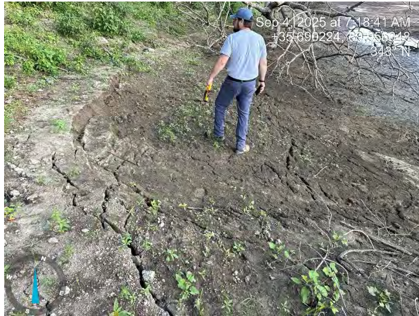
Figure 4: Existing slide on Levee side of proposed harbor expansion
