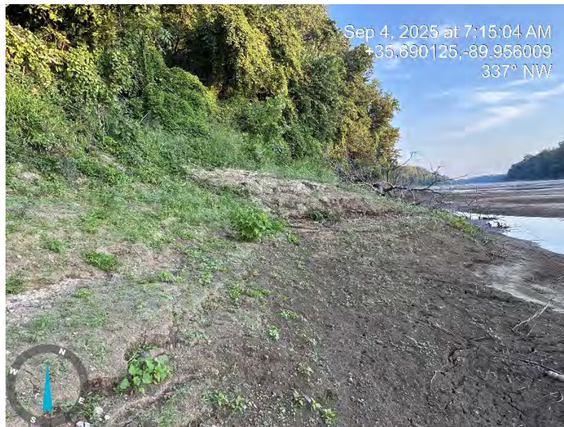
Figure 5: Existing slide on Levee side of proposed harbor expansion
